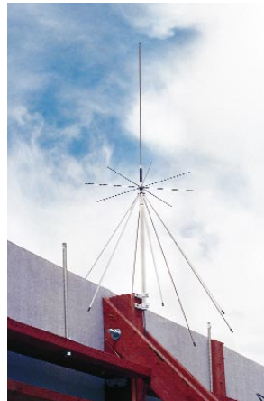
High-gain fixed site VHF antenna
